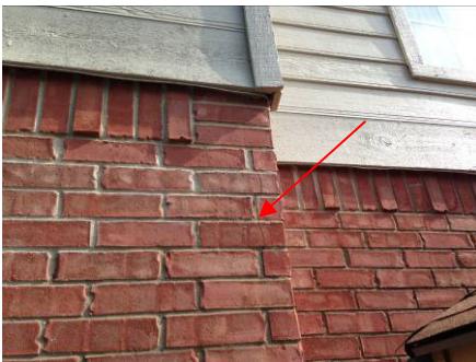
Photos 4 - 8: Minor brickwork separations identified.
