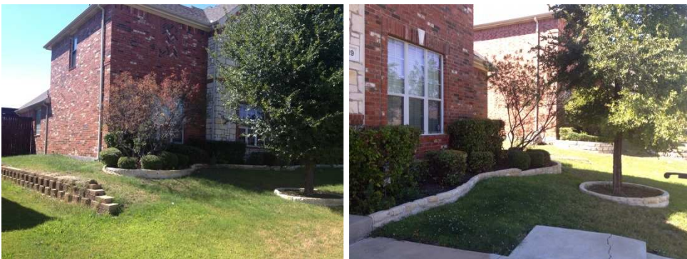
Picture 4 and 5: View of the left and right front of the home. It is hypothesized that there may be fill dirt compaction at the front left corner. This fill dirt compaction, and the large trees, may be contributing to the minor settlement at this corner.
