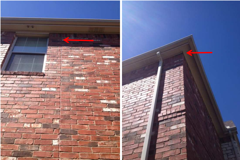
Picture 1 and 2: Indications of minor settlement at the front left corner. Minor expansion joint separation at top and frieze board separation at front left corner.
