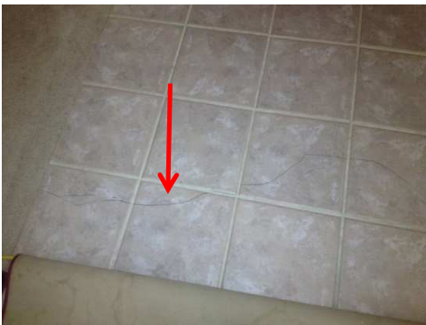
Picture 3: Hairline tile cracking in the front entry, kitchen and master bathroom. These are not indicative of a structural deficiency.
