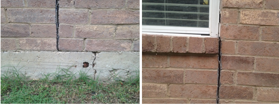
Pictures 3 and 4: Structural slab cracking and distress.
