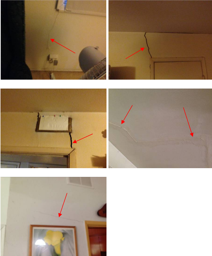
Photos 7 – 15: Drywall separations identified throughout the interior of the home.
