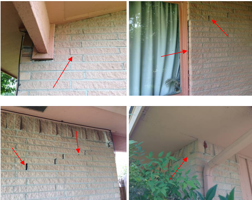
Photos 2 – 5: Brickwork separations and loose bricks identified around the home.
