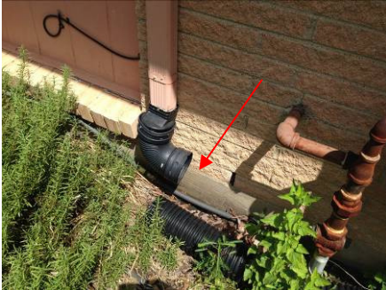
Photo 6: Disconnected gutter downspout along the rear of the home.
