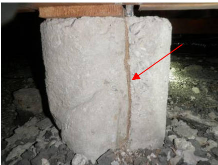
Photo 14: Signs of previous termite activity.
