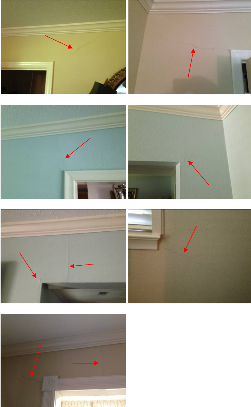
Photos 4 – 10: Minor drywall separations identified throughout the interior of the home.
